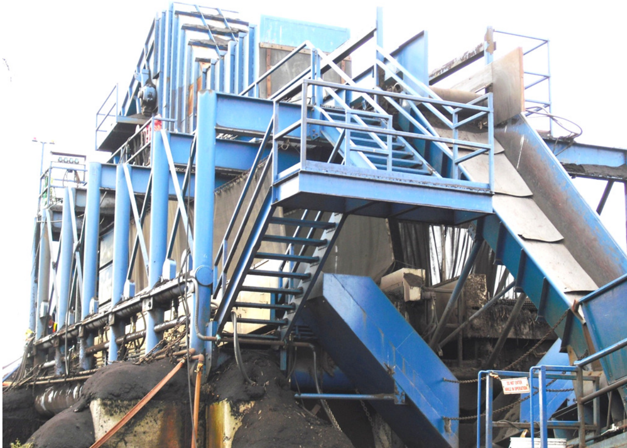
Six-product screening plant - 1,000 CY per hour
