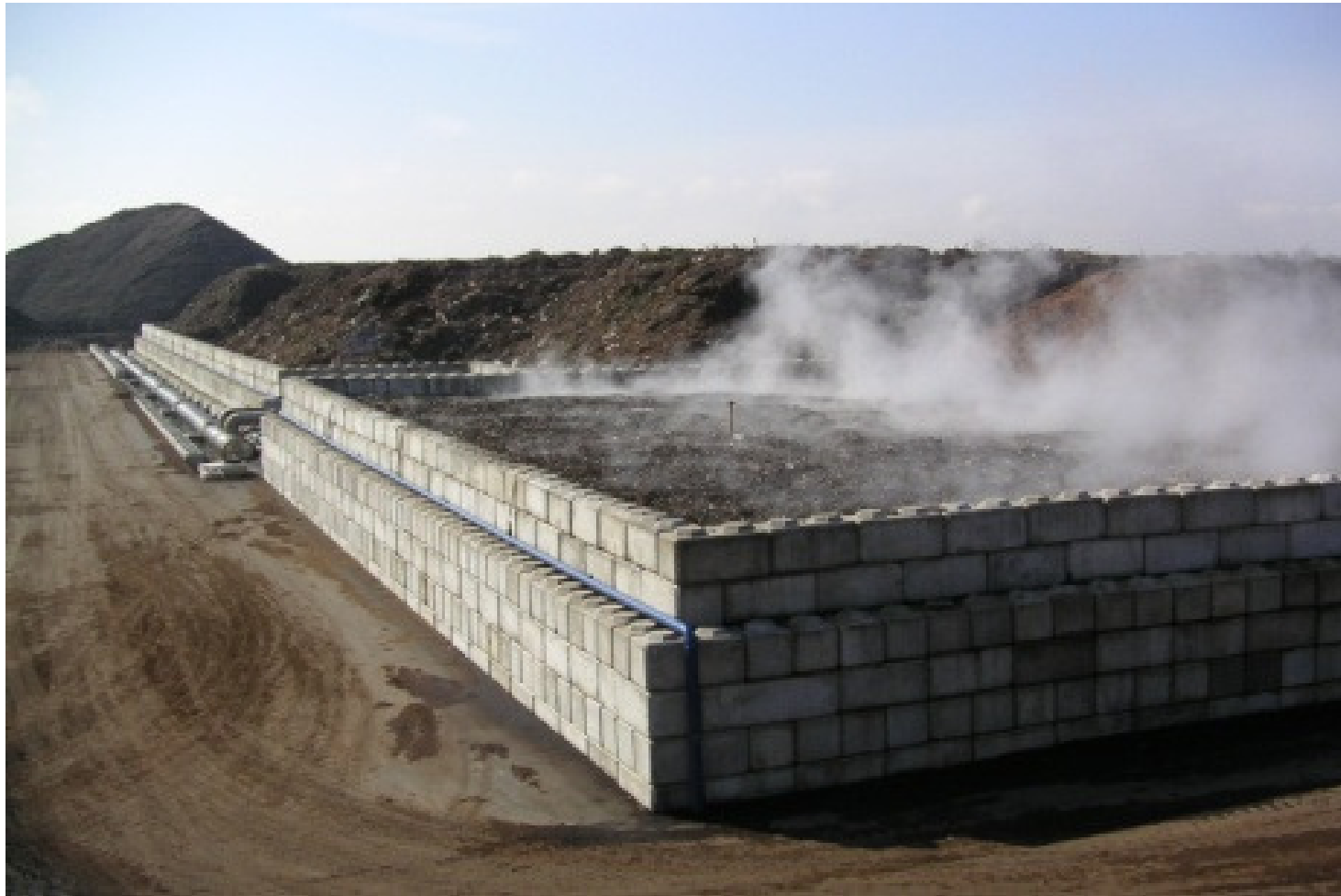
Biofilters - Two at 42,000 cfm flowrate each
