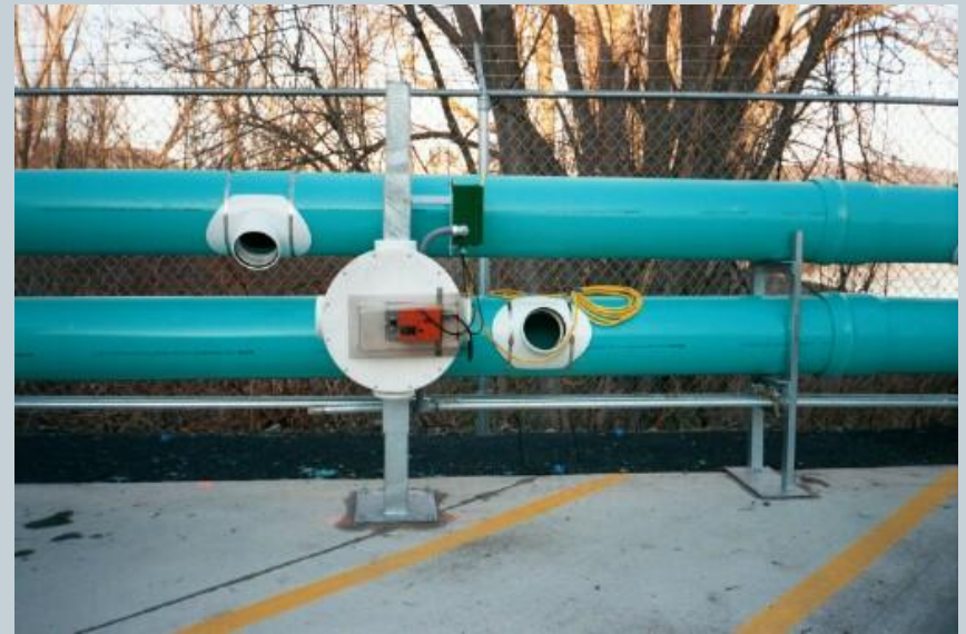
GMT facility in Chenango, NY
