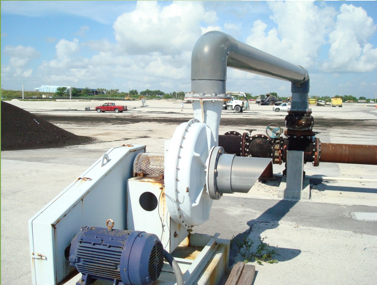
Forced air equipment for aerated static pile.
