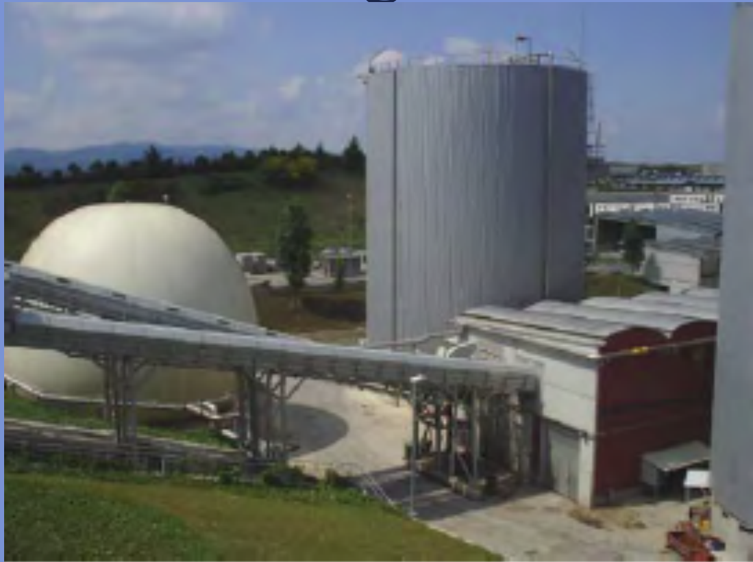
Figure 1 - Anaerobic Digestion Facility, Spain
